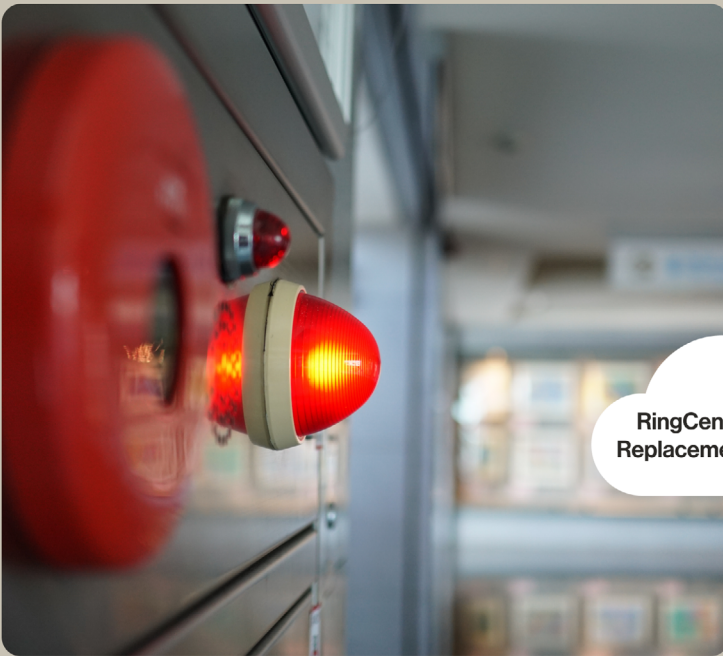
Fire alarm activation
